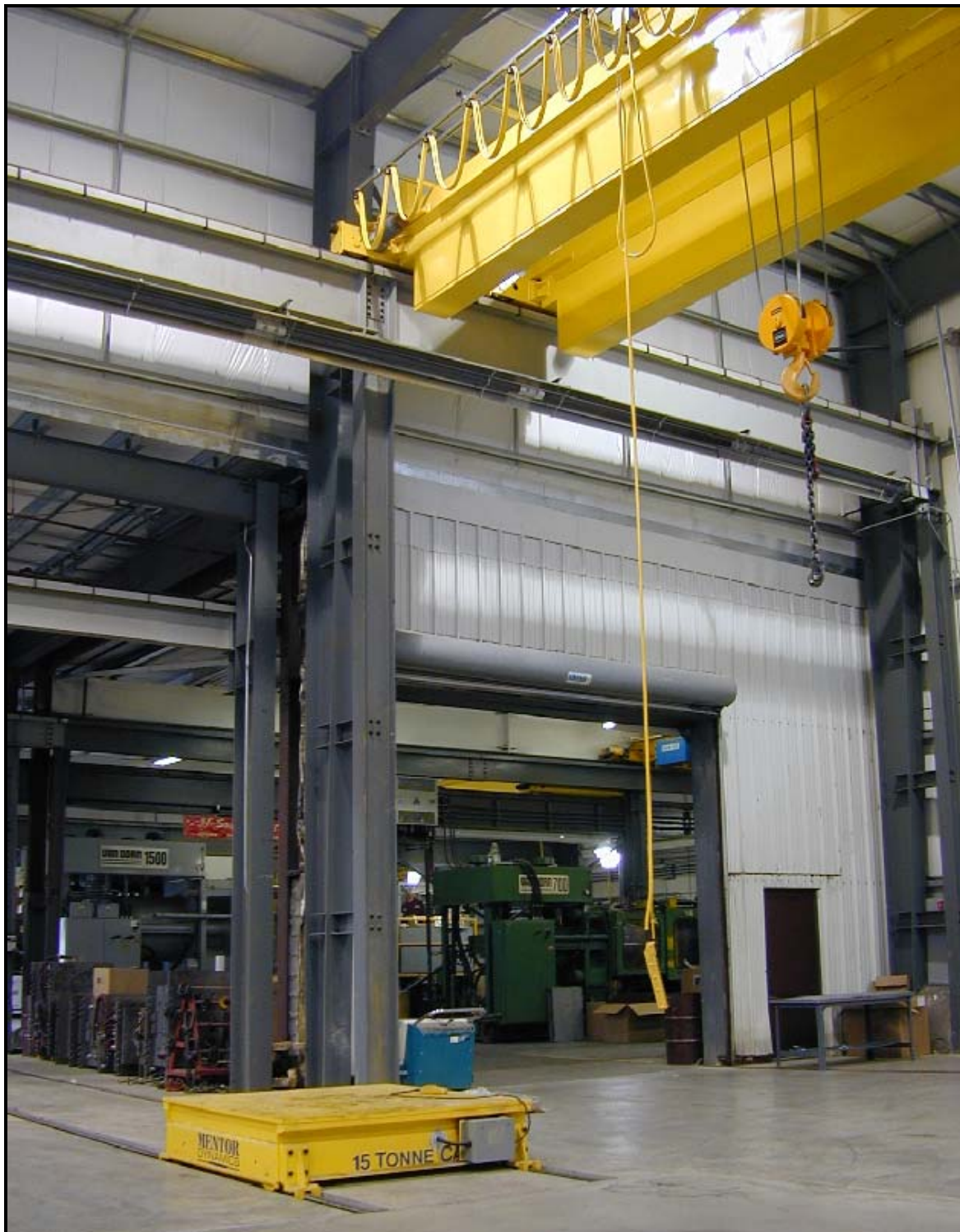
Figure 10-5 – Example of Overhead Crane and Rail-Bound Rail cart Courtesy: Mentor Dynamics
